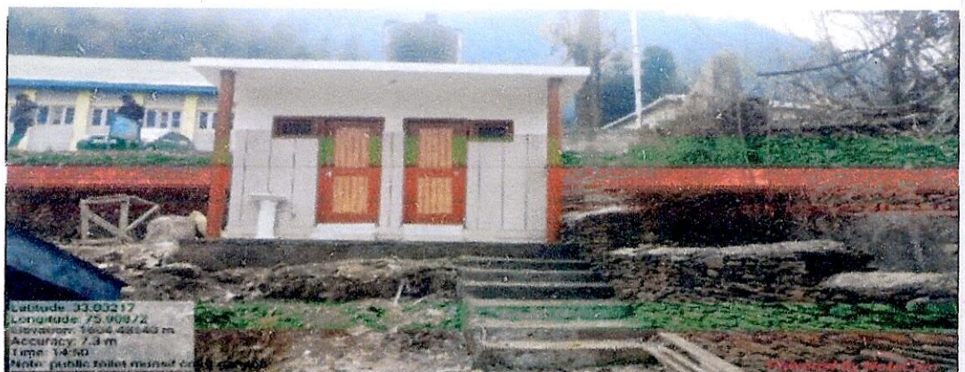
Construction of Common Washroom Block / Public Toilet Blocks (Male / Female) and Reverse Osmosis (ROs) at Munsiff Court Gandoh
